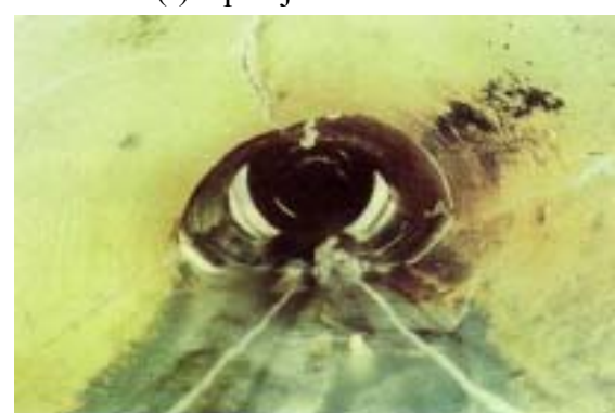
(h) Deformed sewer
