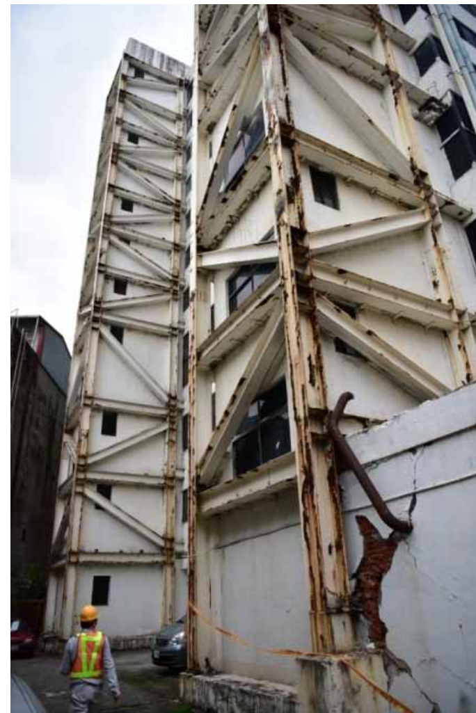
鋼斜撐補強 損壞，未崩塌
